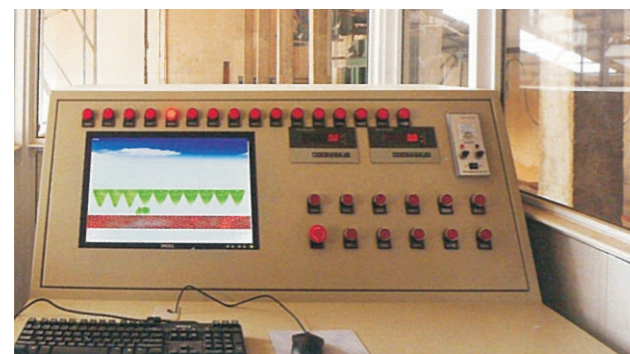
微机配料室 Computer Room ingredients
